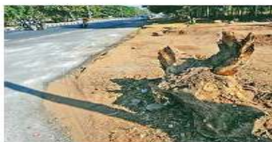
Road widening is going on the 5-km stretch from Sargasan to Mahatma Mandir, venue for Vibrant summit
